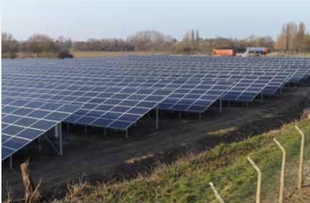
The new solar farm located at London Southend Airport which was built by Stobart Developments.
